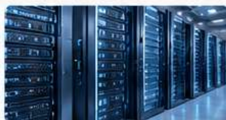
IT & Data Centre Assets Servers, Network Equipment, Racks, UPS
